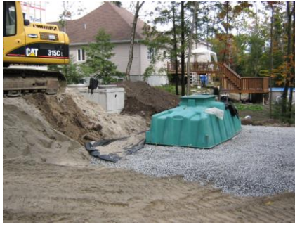
Ecoflo advanced septic treatment system
